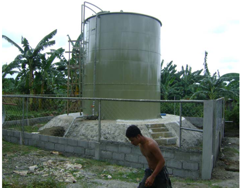
50cum ground level tank of Davao del Sur.
