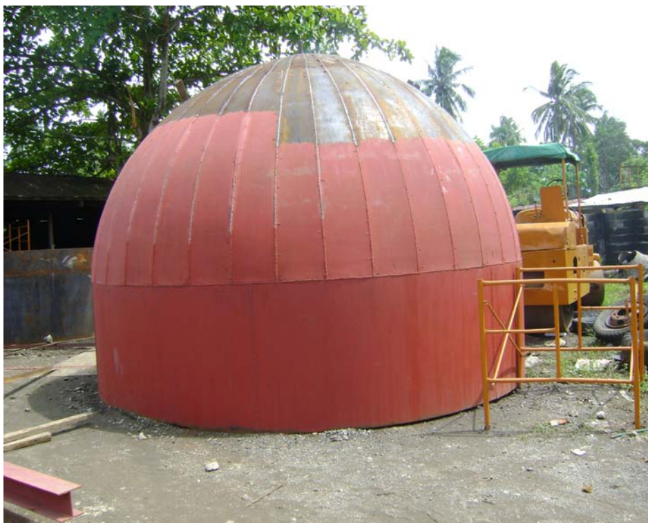
80 cu.m. Elevated Steel Tank of Davao del Norte Project.
